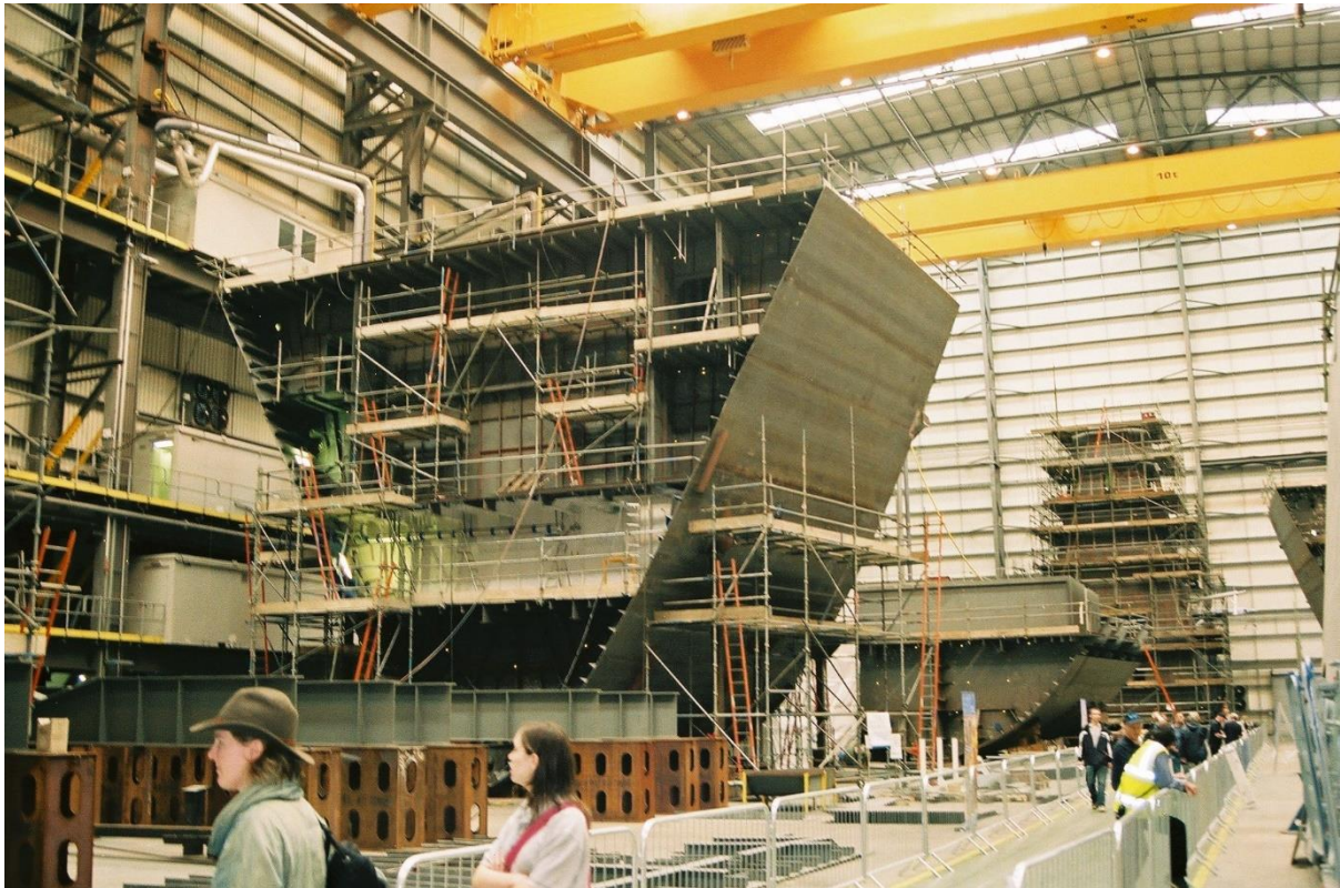
Figure 33. Modular blocks of HMS Dauntless under fabrication at HMNB Portsmouth. Image courtesy Adrian Jones.
